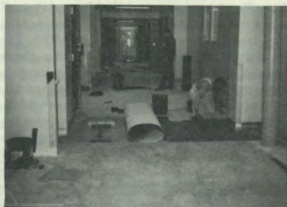
◀ Construction on both the new basic science building and the addition to the Medical School Hospital is expected to be completed in March of 1972, according to A. J. Clemons, director of facilities planning.
