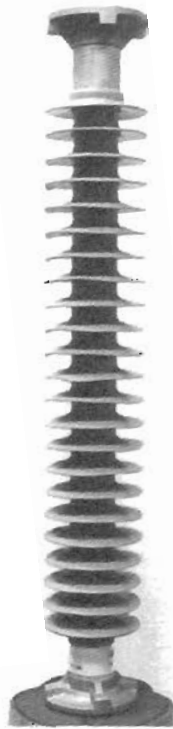
Figure 1.4 : Substation insulators: (a) Porcelain insulators in service, and (b) Typical 115 kV composite substation insulator.
